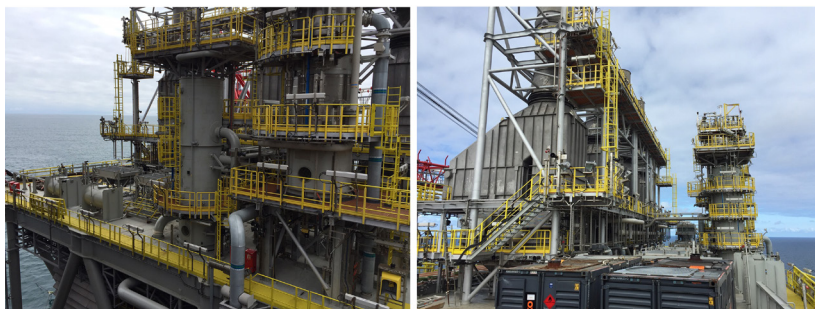
Figure 2. Almost 2.6 miles of the MARRS® OFFSHORE handrail system was installed throughout the entire Clair Ridge facility. The handrail system meets strict NORSOK safety requirements and is dramatically more corrosion resistant than steel.
