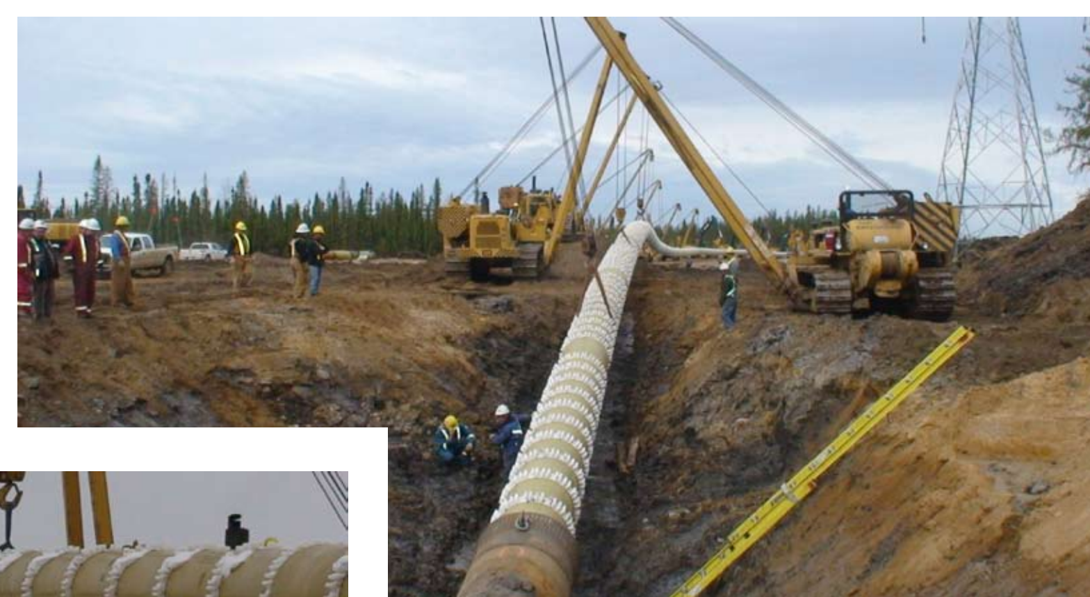
Twenty-five pieces of equipment (19 side booms and 6 excavators) handled the entrance side of the bore while the drill rig pulled from the exit side
