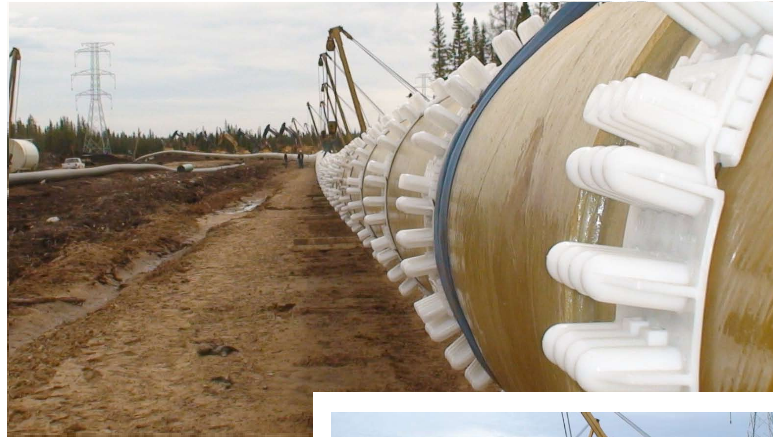
36" diameter GRE pipe. The white casing spacers protect and centre the GRE as it is pulled through the 48" diameter casing pipe already inserted into the previously drilled 60" diameter HDD bore
