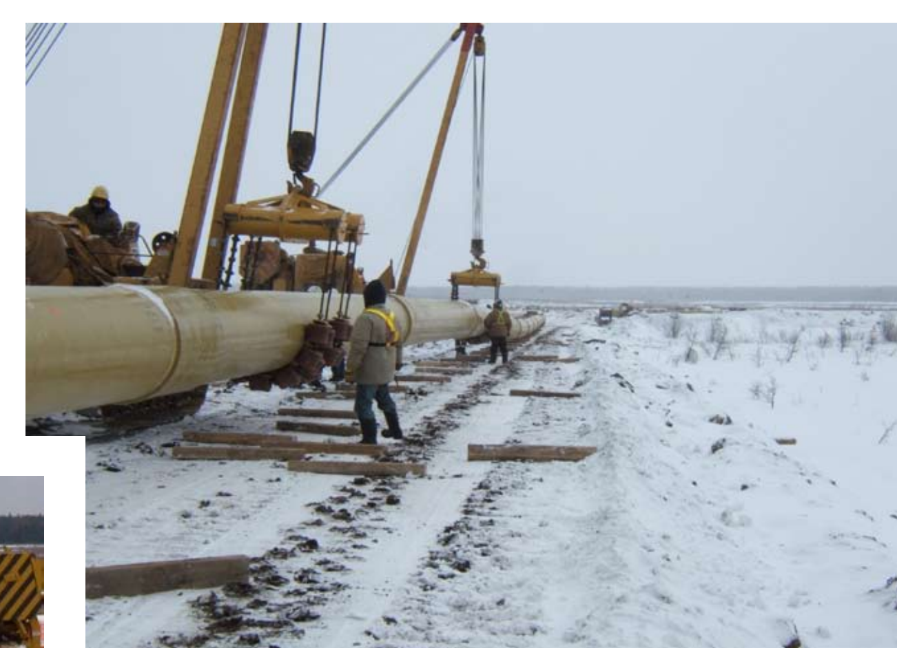
Right of Way Stringing Many aspects of the installation of the fibreglass pipeline are logistically challenging including extreme cold weather, muskeg conditions, and limitations on bending and pulling stress.
